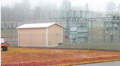
Electrical Equipment - Sub Station Enclosure
